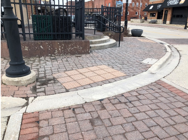
The use of concrete detectable warnings and bricks in the crosswalks and sidewalks provide irregular surfaces that are potential tripping hazards.
